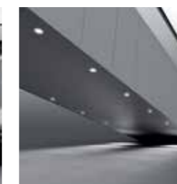
Soffit LED spot cladding lighting
